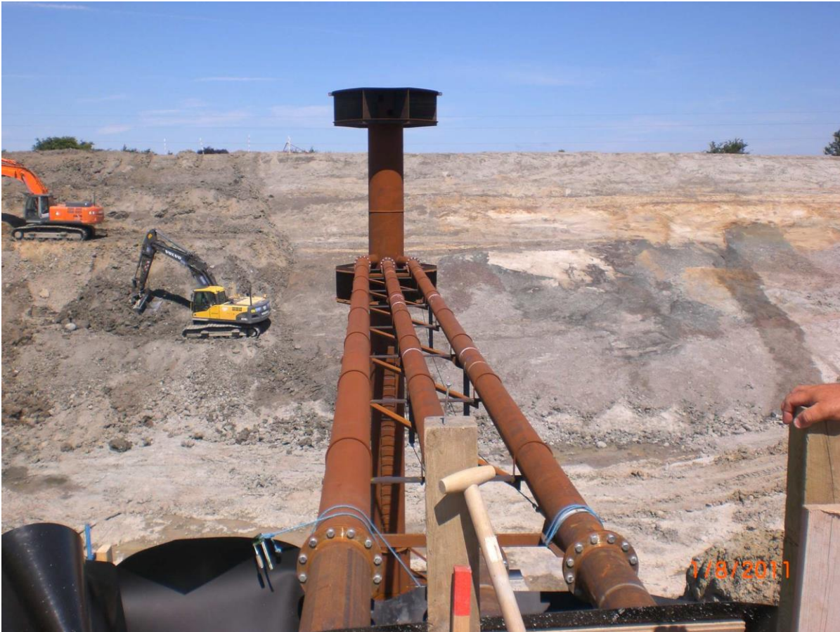
Figure 13. In-/outlet arrangement led through the side of the storage. Photo from the implementation of the SUNSTORE 4 storage in Marstal.
