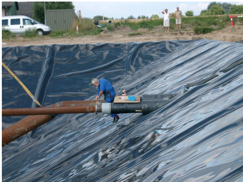
Figure 22 Inlet and outlet pipes. The leak was in the liner weld during one of the pipes [10].
