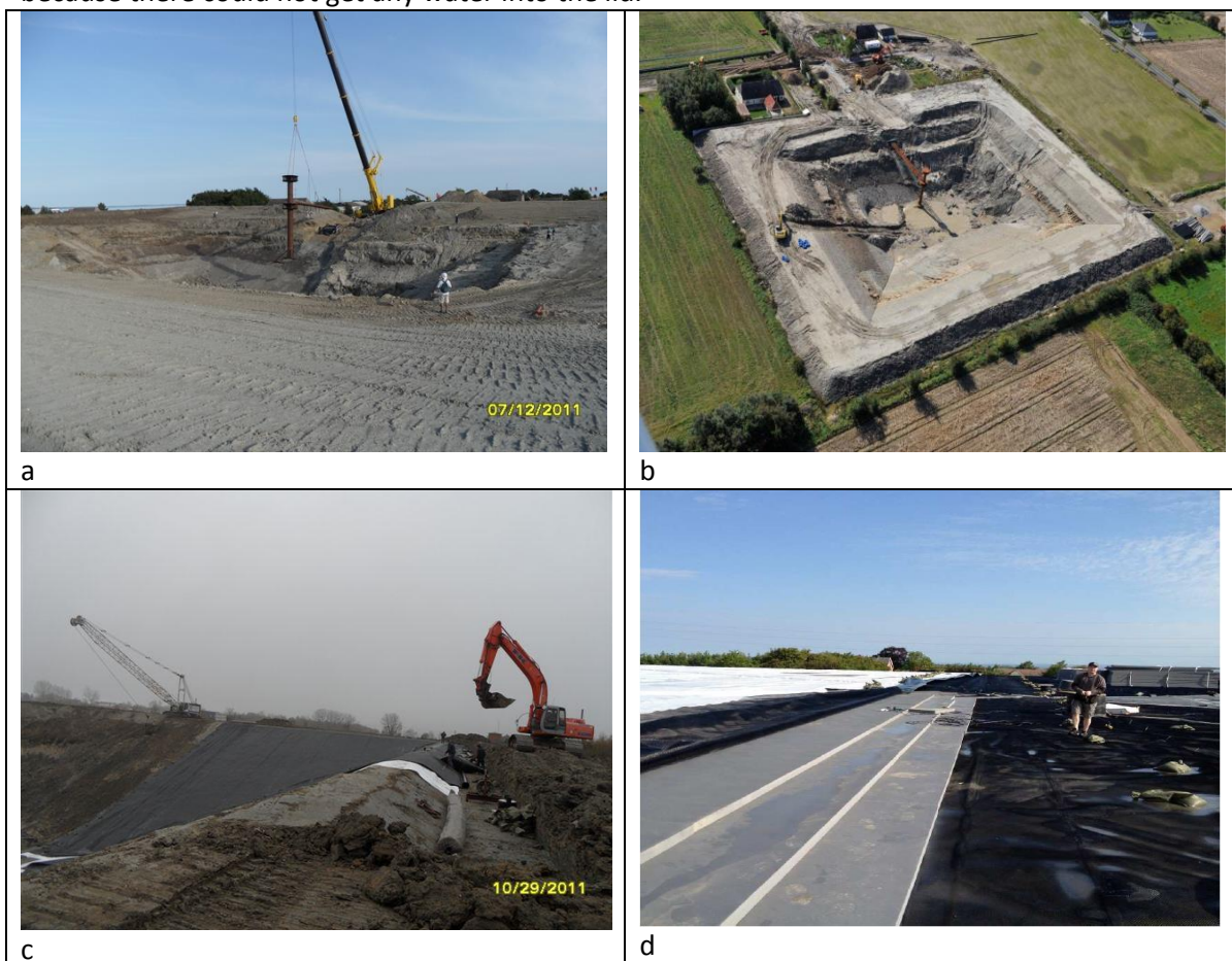
Figure 25 Figure 2.2.11: Construction of the storage in Marstal [13]. a: inlet and outlet pipes are hoisted into place. b: the storage after the cloudburst. c: The liner work. d: the lid is built.
